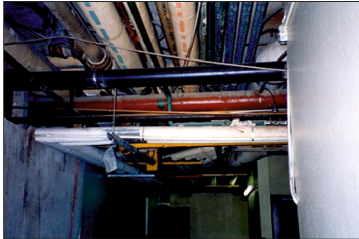
Figure 2.1a Earthquake Hazard of Electrical Conduits (Images from Federal Emergency management Agency Website, www.fema.gov )
